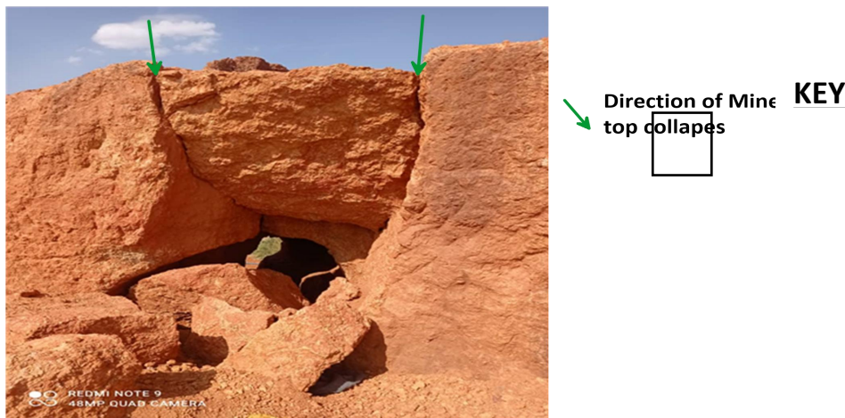
Figure 11. Guratopp Mine Site- Typical Mine Rooftop Collapse along the Mine Tunnels
