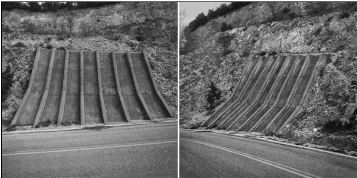
Fig. 1 A concrete retaining wall in the Aliakmon River area, West Macedonia, Greece, having buttresses with varying slope [17]
