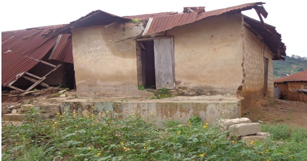
Figure 4: Building that fall with 1km radius damaged by the effects of stone blasting in Akure-Ado axis
